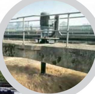
Deck mounted "splash" aerator
